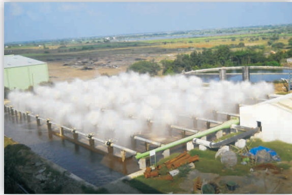
Advance Mist Cooling System.
